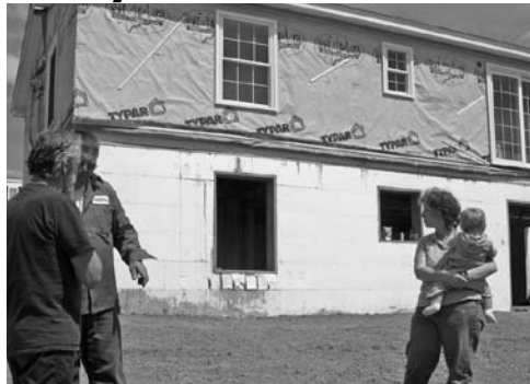
NMCC residential construction instructor Guy Jackson (left) talks with homeowners Kevin and Holly Tompkins, with daughter Sadie, as their new home is placed on its foundation.
