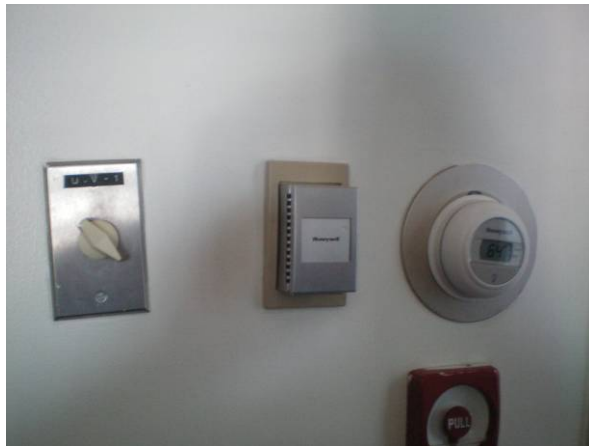
Snow Unit Ventilator Control
