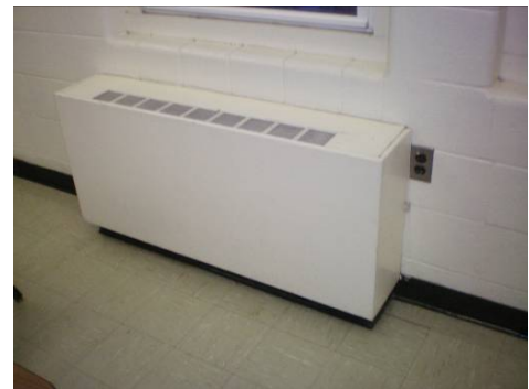
Old Unit Ventilator Converted to Fan Coil
