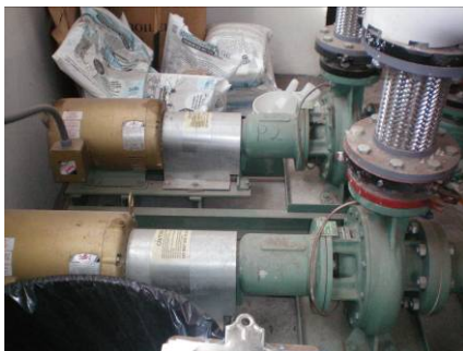
Building Heating Hot Water Pumps
