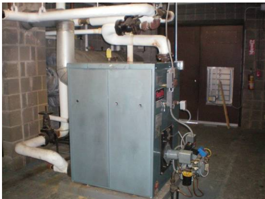
Existing Washington Hot Water Boiler
