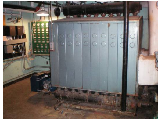
Existing Andrews Hall Boiler
