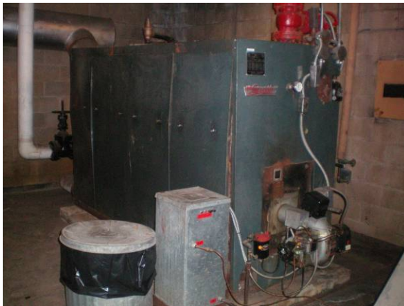
Existing Hot Water Boiler
