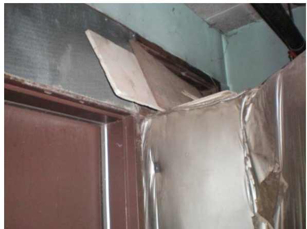
Outside Air Intake Covered Over
