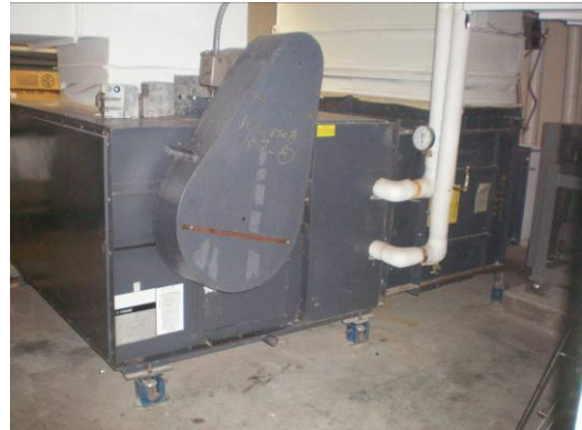
Electronics Lab Heating and Ventilating Unit
