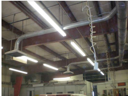
Ductwork to Auto Body Smokeeater
