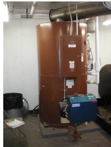
Snow Domestic Hot Water
