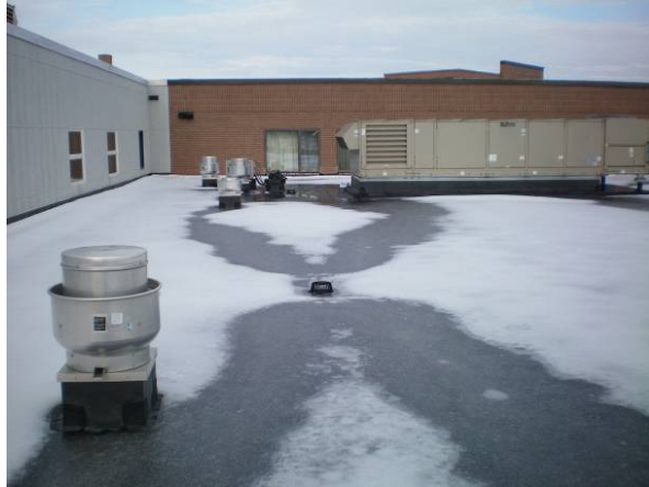
RTU-1 Library Air Handler
