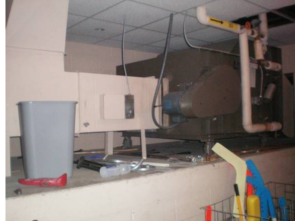
Women's Locker Room HV Unit
