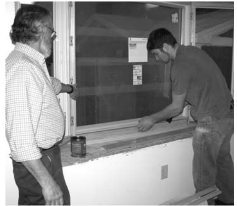
Residential construction instructor Guy Jackson (left) provides guidance to senior Brandon Smith as he does some of the finish work around a window on house #31.
