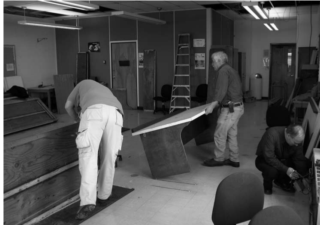
Work has begun on renovating the future MMG Insurance Classroom at NMCC, which will transform Christie 208 into a modern business environment similar to what is found at MMG. The project is expected to be completed this summer. Removing the old furnishings and preparing the room for the renovation work are (left to right) NMCC employees Robert Smith, Steve Caron and Barry Ingraham.
