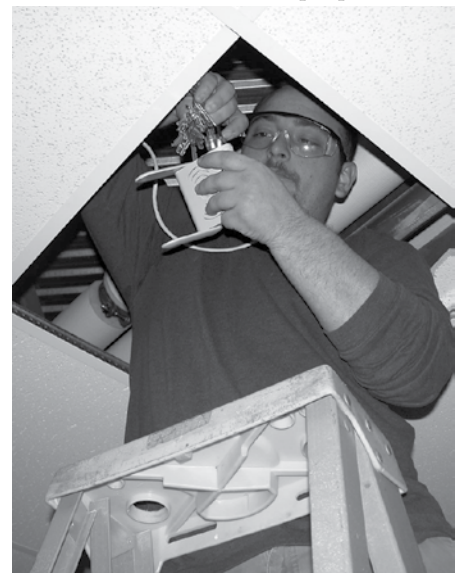
Shawn Lahey, from the College’s IT department, installs one of the wireless access points on campus, made possible through the donation from Katahdin Trust Company.
