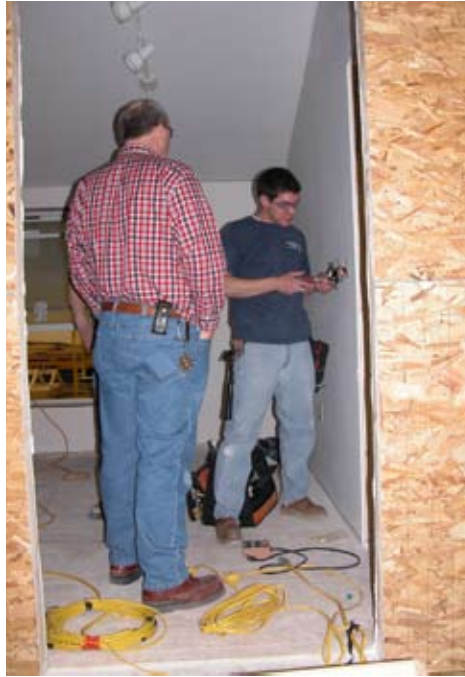
NMCC electrical construction and maintenance instructor Charles Kelley observes Jan Perreault, a student in his program, as he works on a light switch in the 30th home built by the College for the Sinawik project.
