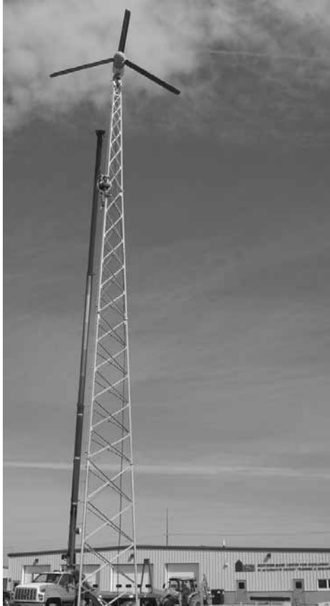
Crews from Northern Electric Incorporated of Ashland install an 80 foot tall residential wind turbine at the site of NMCC's alternative energy center.
