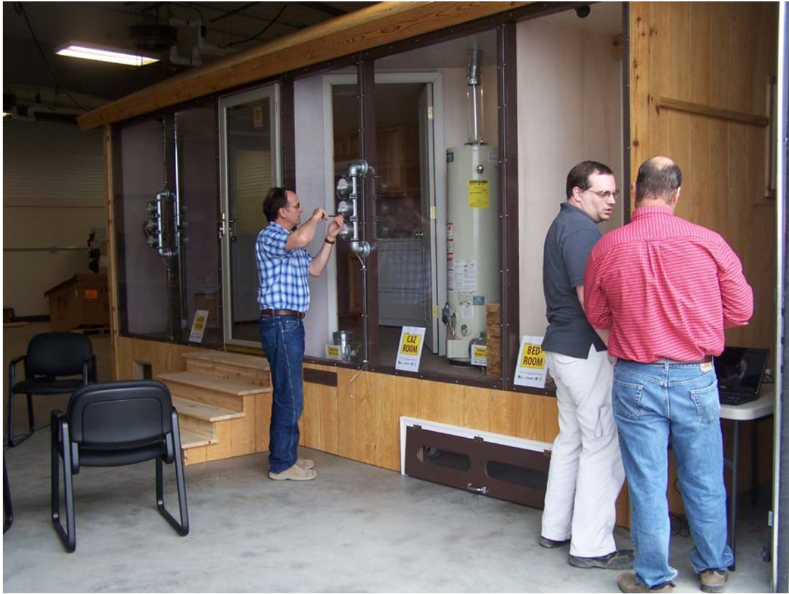
Northern Maine Community College plumbing and heating instructor Alan St. Peter (left) along with Robert Smith, NMCC information systems support specialist (center) and Todd Maynard, NMCC electrical construction and maintenance instructor work on the newly installed pressure house in Maine's newest Weatherization Training Center in NMCC's Northern Maine Center for Excellence in Alternative Energy Training and Education at 920 Skyway Street on the Skyway Industrial Park in Presque Isle. A community open house for the center is planned for this coming Thursday, October 27, which has been proclaimed Maine Weatherization Day.
