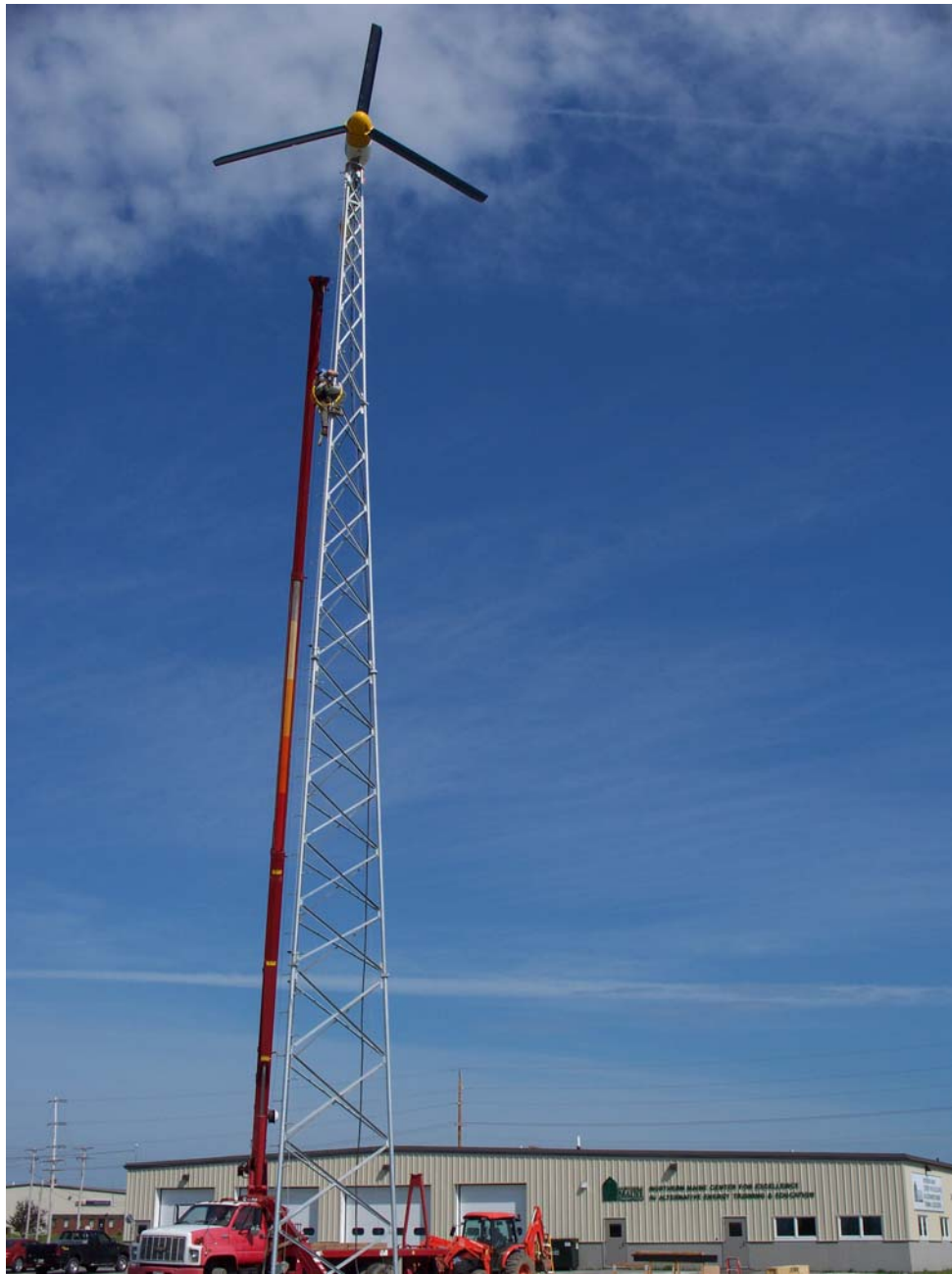
Crews from Northern Electric Incorporated of Ashland install an 80 foot tall residential wind turbine at the site of Northern Maine Community College's Northern Maine Center for Excellence in Alternative Energy Training and Education.
