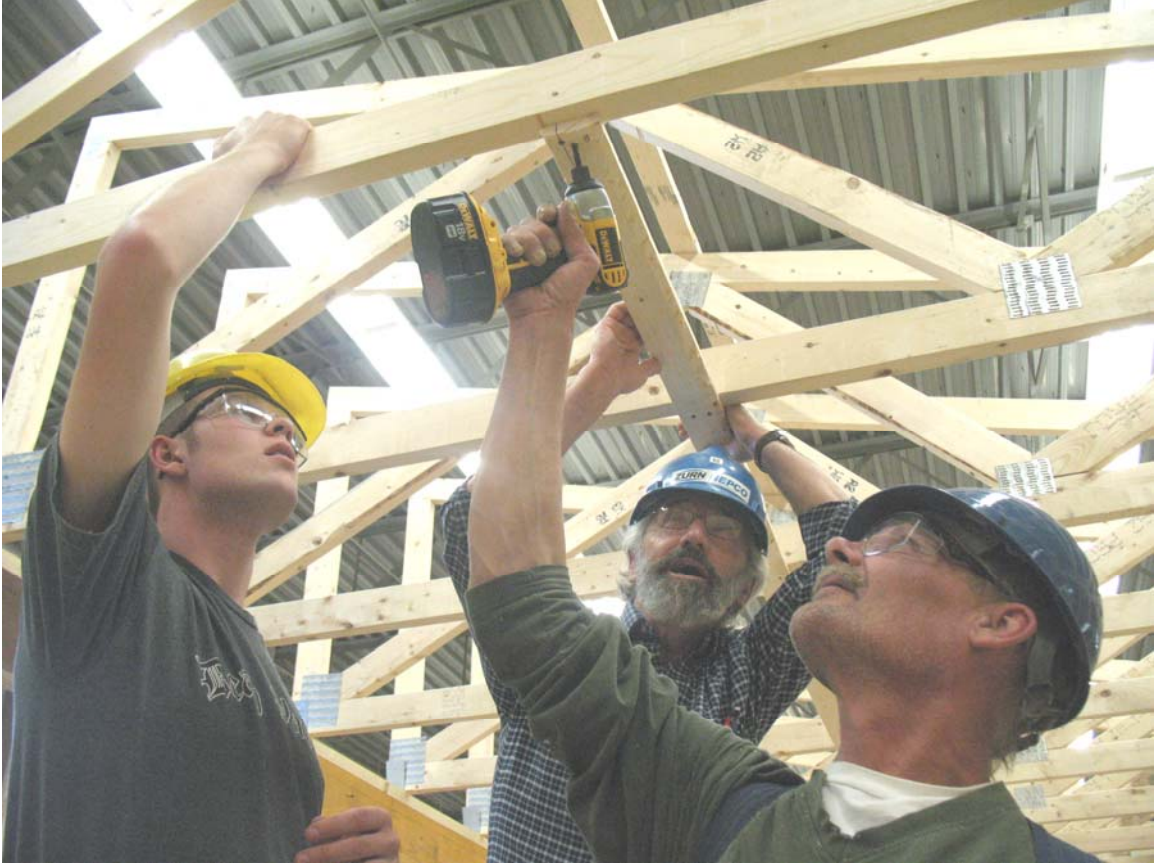
Northern Maine Community College residential construction instructor Guy Jackson (center) works with first year students John Dumond of Cyr Plantation (left) and Jon Sund of Stockholm (right) on the framing work of Sinawik house number 33 in the residential construction lab at the College.
